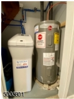
Water softener and heater
