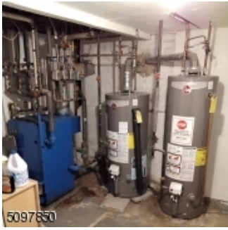
1 Unit, Separate Water Heaters
