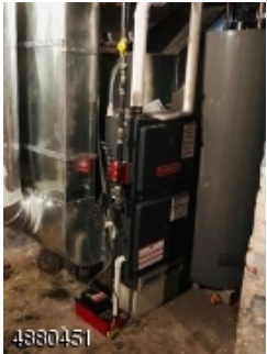
Identical Boilers all units
