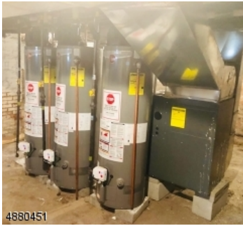
Hot Water Heaters
