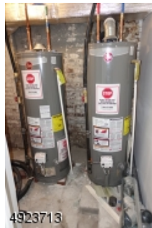
Hot Water Heaters
