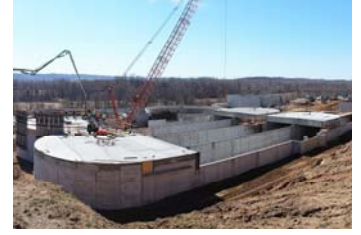
Wastewater Liberty Wastewater Treatment Plant Liberty, MO
