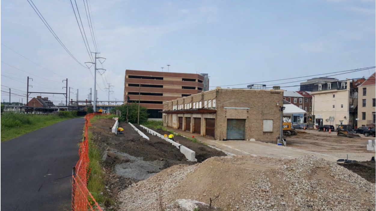
Schuylkill River Trail and south side of building during construction of retaining walls.
