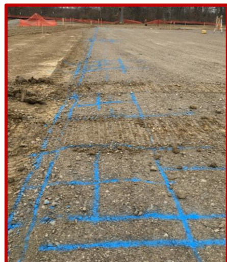
Picture 3: Layout of foundation in Area H, the future location of Early Childhood Development
