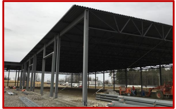
Picture 1: Structural steel in Area C, the future location of Auto Tech, Alignment, & Collision
