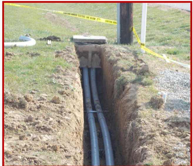
Picture 2: Underground conduits for fiber optic
