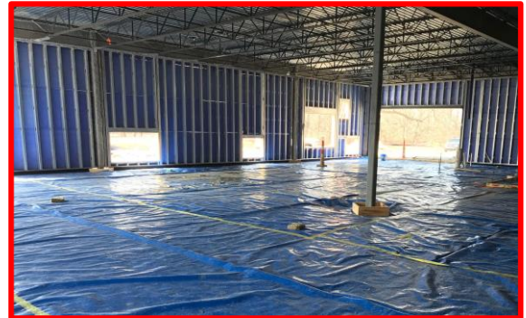
Picture 2: Preparation for Slab on Grade pour in Early Childhood Development Area
