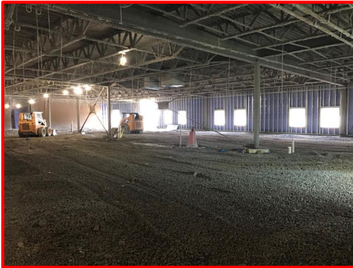
Picture 4: Prep for Slab on Grade Placement in the East Admin Area
