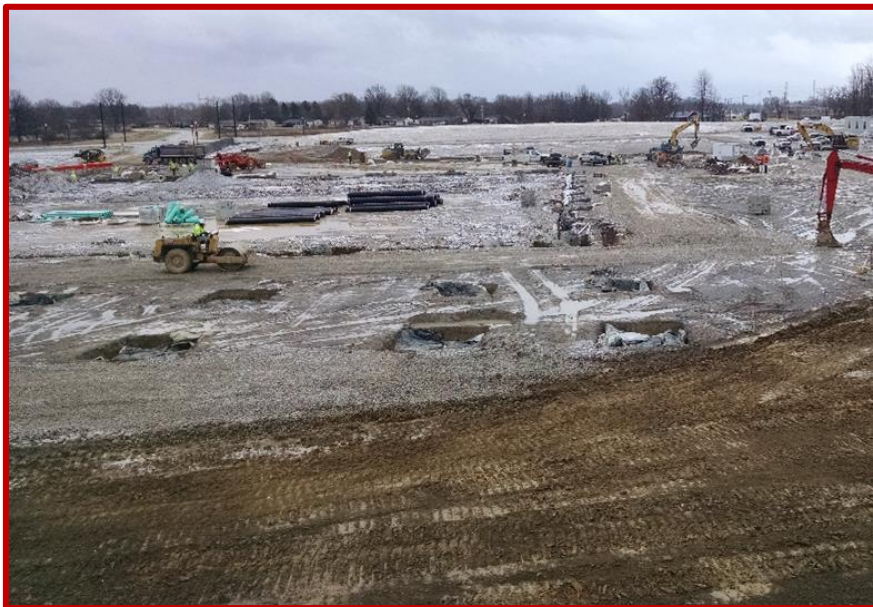
Picture 5: Site progress of the building pad and foundations on south side of campus
