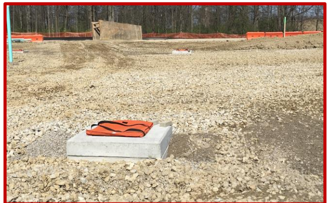
Picture 3: New storm structures in the service yard/courtyard between Areas A and E
