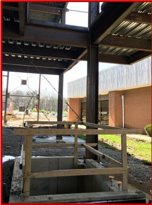
Picture 4: Area D's second floor structural steel making way for the elevator shaft below
