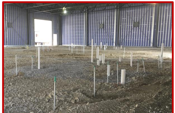
Picture 3: Progress of underground electric and completed underground plumbing in Area A
