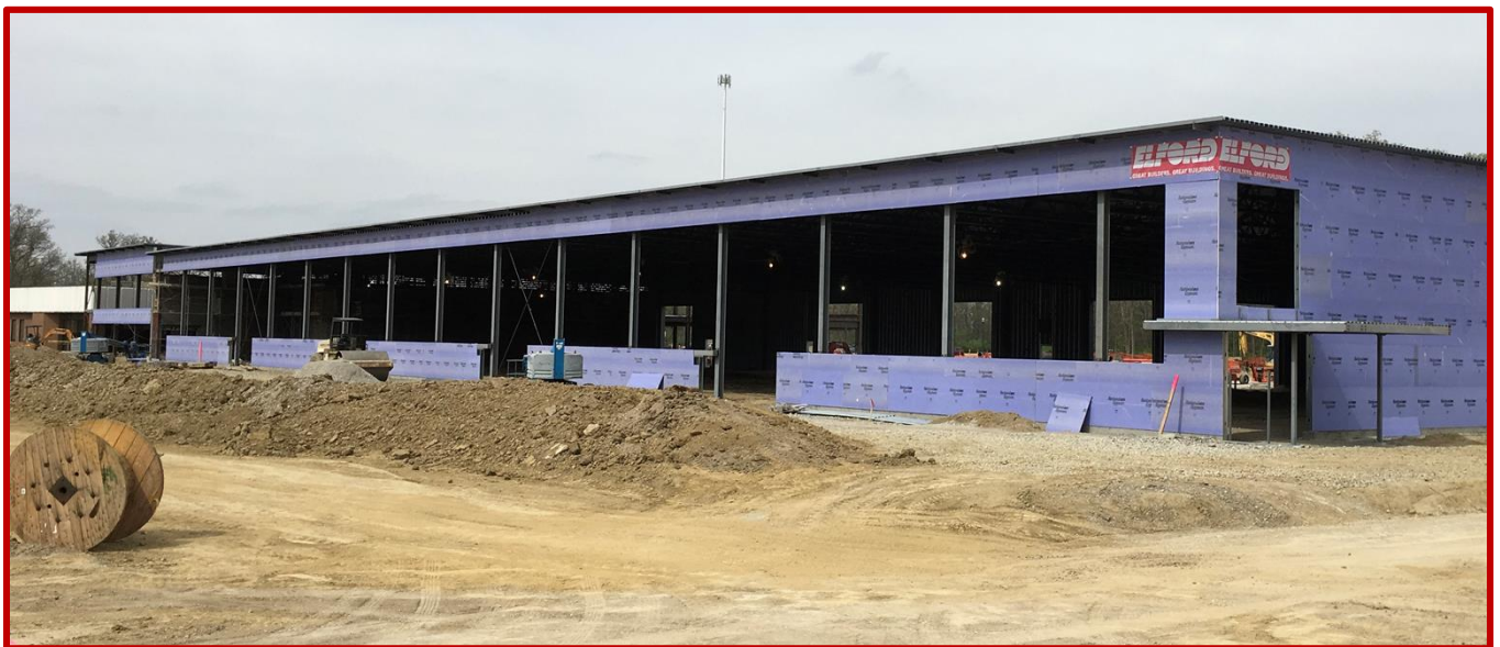
Picture 6: Metal framing and exterior sheathing progress on the West side of Areas B, C, and D
