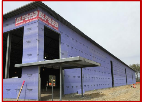
Picture 1: Sheathing at the South West corner of Area B's entrance canopy
