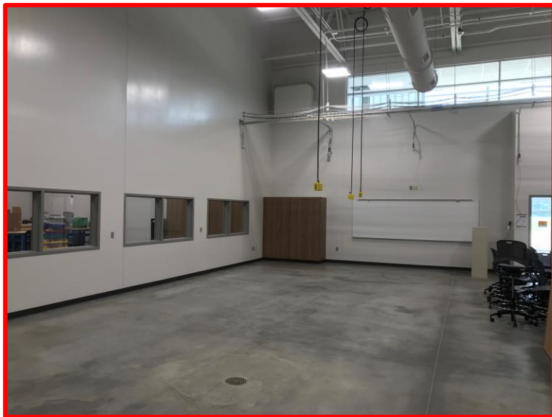
Picture 5: Electrical Drops in Engineering Tech High Bay Lab
