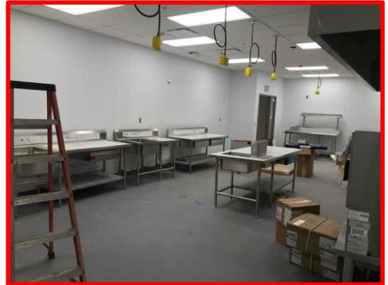
Picture 1: Kitchen Equipment in the Professional Food Service Kitchen
