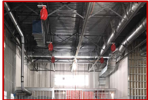
Picture 1: Hose Reels installed at the Engineering Tech. Lab
