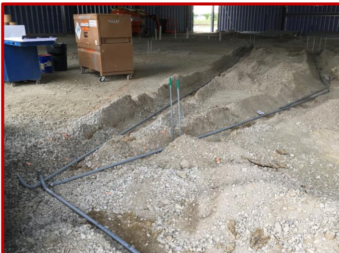
Picture 6: Underground electrical conduit runs in Area A labs
