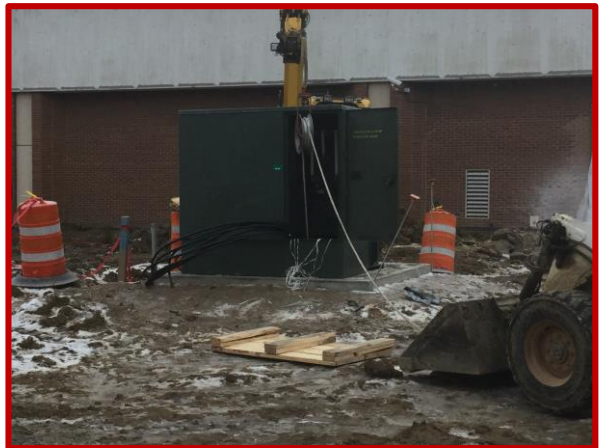
Picture 2: Transformer installed by AEP
