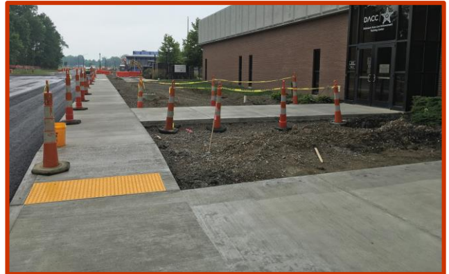
Picture 2: New sidewalks and ramps outside of the main entrance and Law Enforcement training
