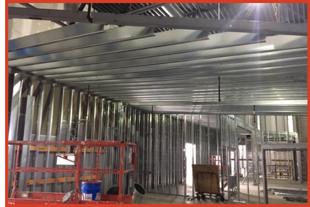
Picture 1: Interior Framing of Shared Classroom for Auto Body and Power Sports and Diesel
