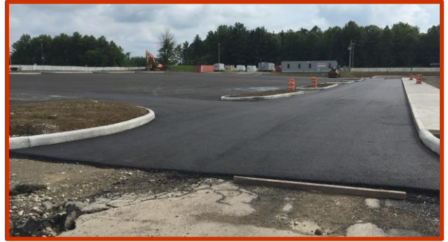
Picture 1: The base course of asphalt at the entrance of the South parking lot
