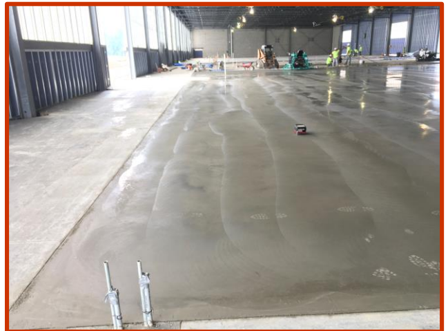
Picture 2: Newly placed concrete slab on grade in Area B being tested for floor flatness/floor levelness
