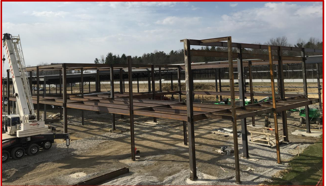
Picture 4: Progress in Areas D and E as steel beams make way for Digital Design and Application Development on the second floor
