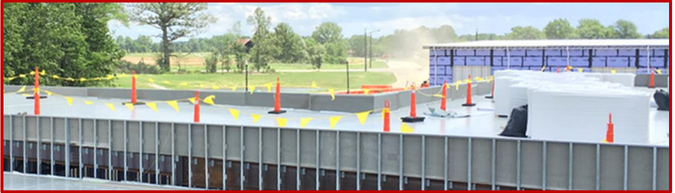
Picture 4: Progress of parapet walls and roofing atop Area E's new LGIA
