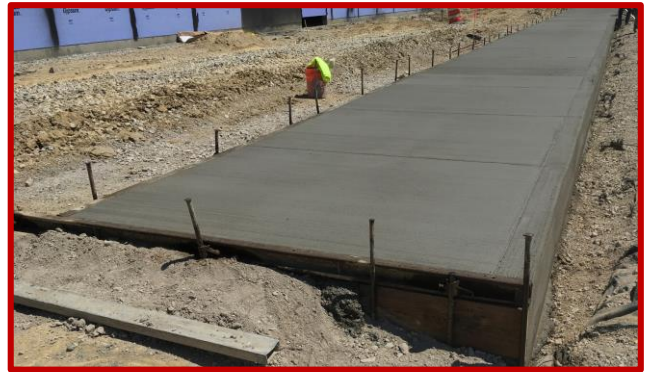
Picture 1: Curing sidewalk along Areas A and B in the South parking lot
