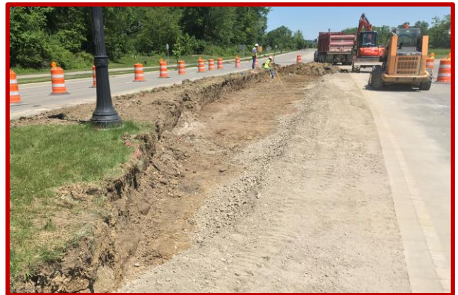
Picture 2: Excavation into the existing center island for the Glenn Parkway turn lane into campus
