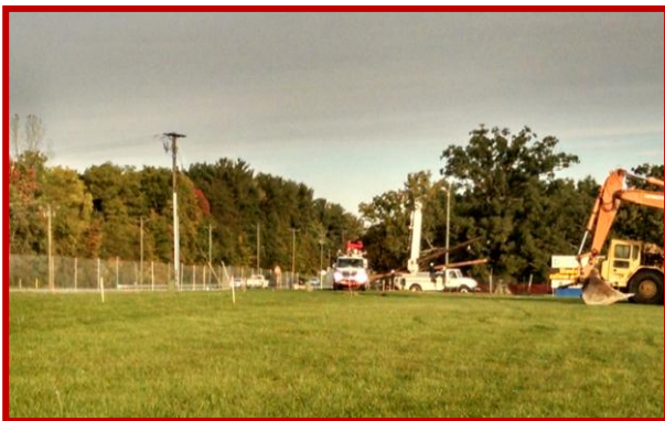
Picture 2: Temporary power for site
