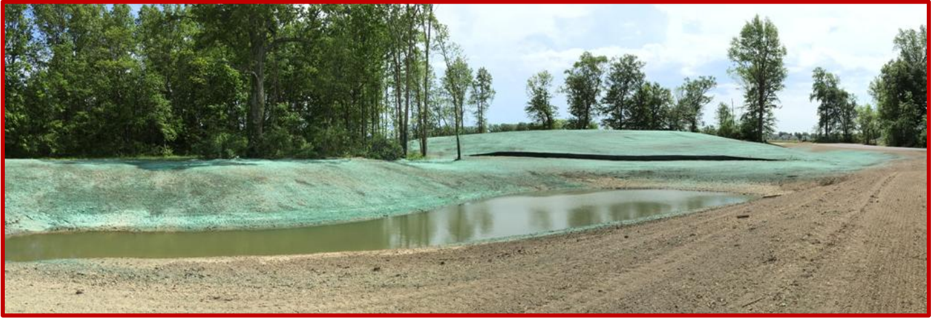
Picture 4: The beginnings of hydromulch seeding at the retention bond behind the future Burn Building
