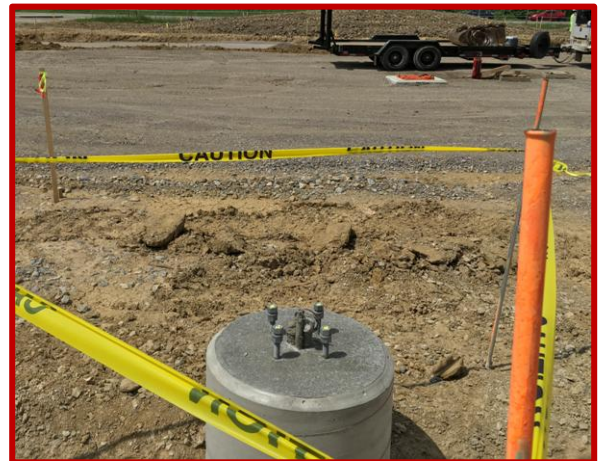
Picture 2: Newly installed light pole base at the North West parking lot
