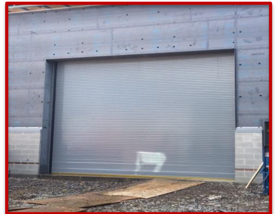
Picture 1: Overhead Coiling Door at Welding Area
