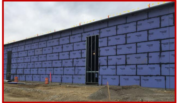
Picture 1: Caulked sheathing and metal framing for window enclosures in Area A
