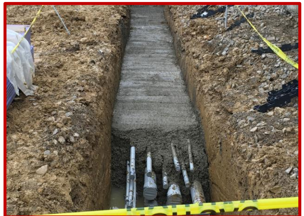
Picture 3: Newly placed concrete encasing electrical conduit in the courtyard along Area E South
