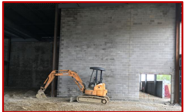
Picture 2: The completed masonry firewall between Power Sports & Diesel and Student Dining
