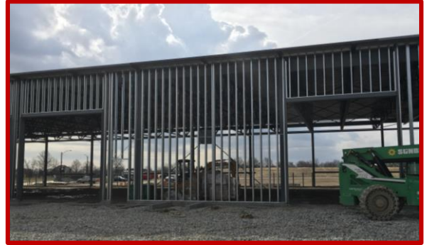
Picture 1: The start of metal stud framing on the north side of Area A
