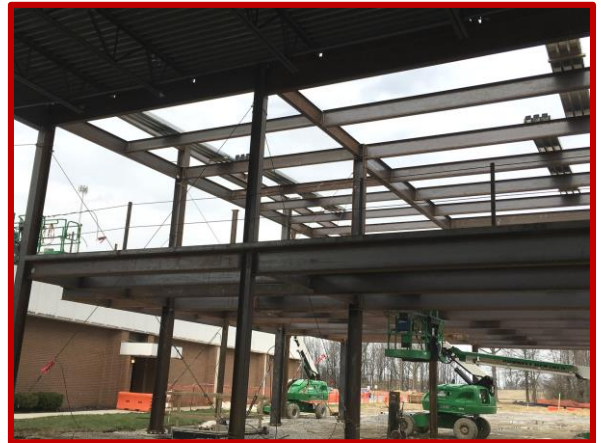
Picture 2: Metal decking and the second floor railing progress in Area D
