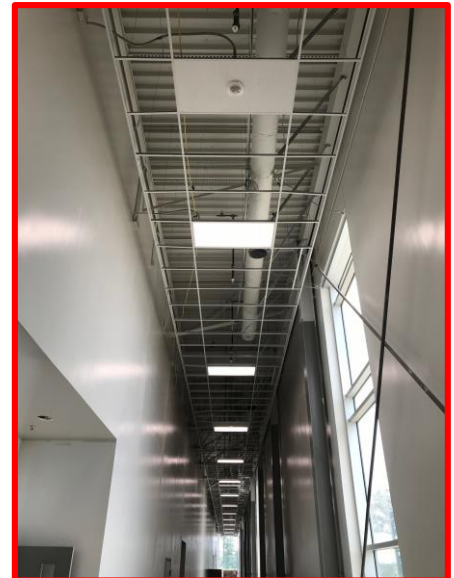
Picture 3: Lighting and Fire Alarm Devices in the North-South High Bay Lab Corridor
