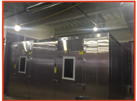
Picture 2: Walk-in cooler Installed in Culinary Arts Kitchen
