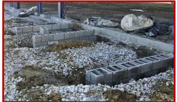
Picture 2: Finishing the masonry foundation for the service canopy outside of Welding Labs
