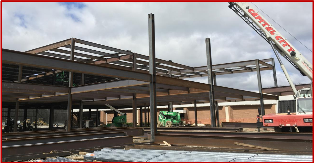
Picture 5: Structural steel progress for Hospitality, Landscape, and Culinary Arts in Area E
