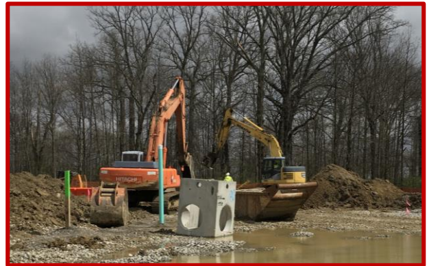
Picture 2: Excavation and installation of storm structures in the courtyard between Areas A and E
