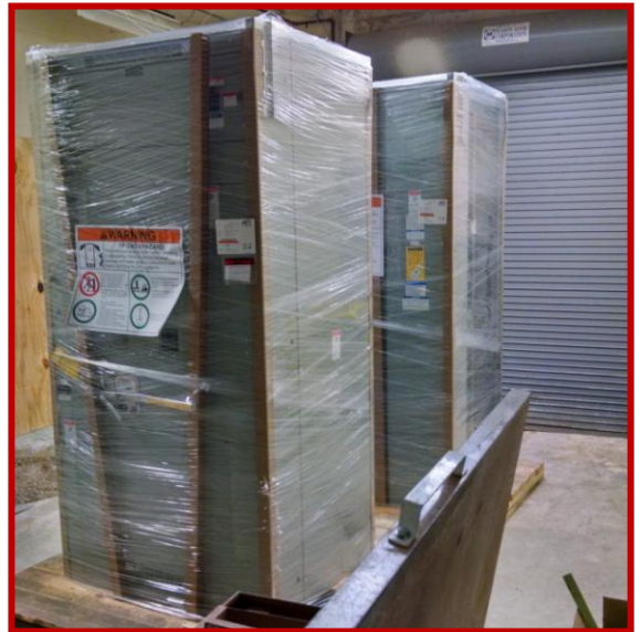
Picture 1: Switchgear delivered to the site
