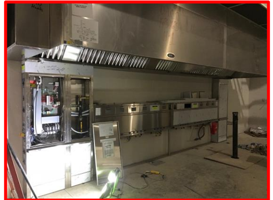
Picture 2: Energy Distribution System in the Main Kitchen
