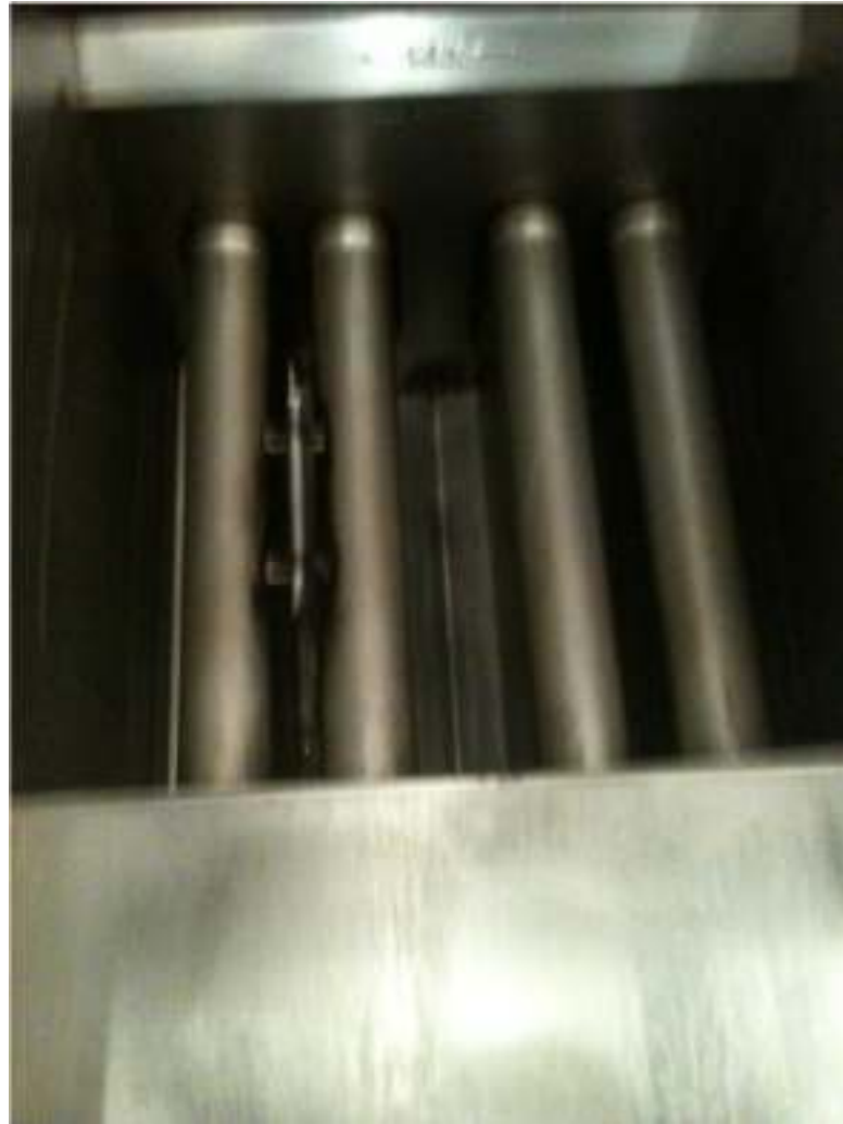
After FiltaFry Cleaning
