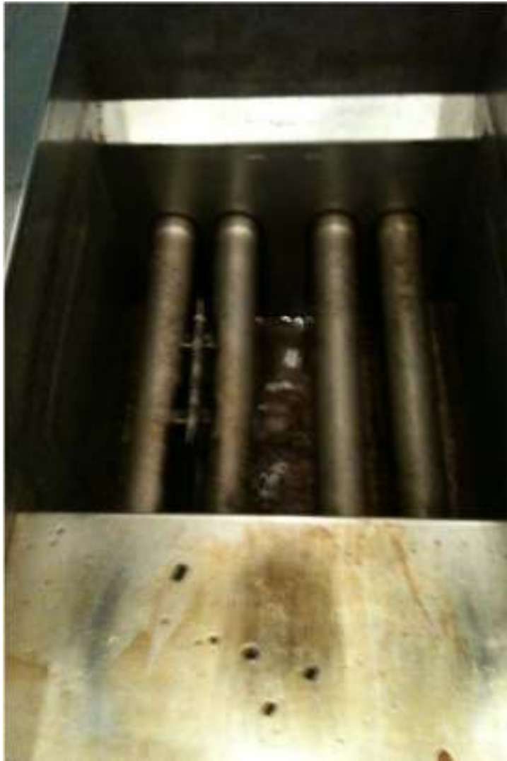
Before FiltaFry Cleaning
